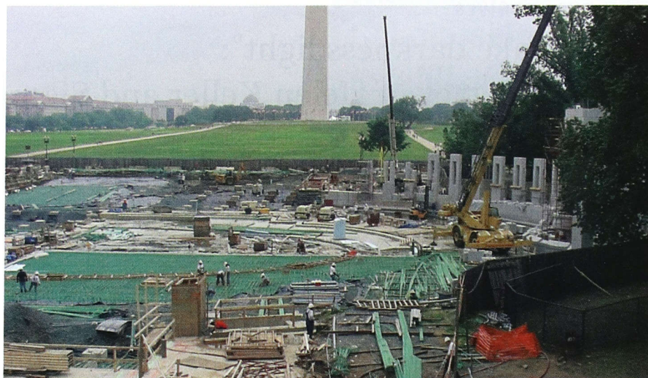
This view of the south end of the memorial plaza shows the rebuilding of the Rainbow Pool (center) with the Washington Monument and Capitol in the background.
